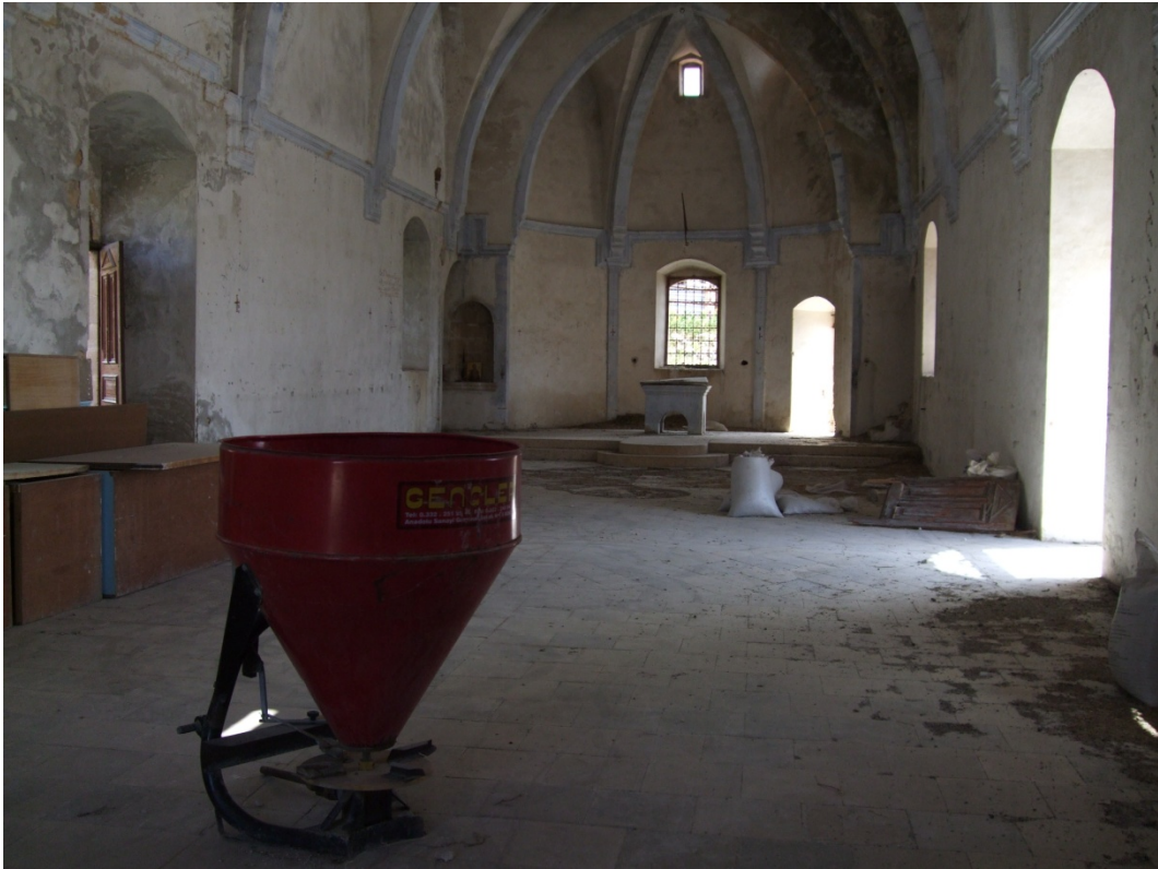
Figure 21: the gutted interior of the Church of Agios Gordios(?) in Agridaki/Alemdağ.
